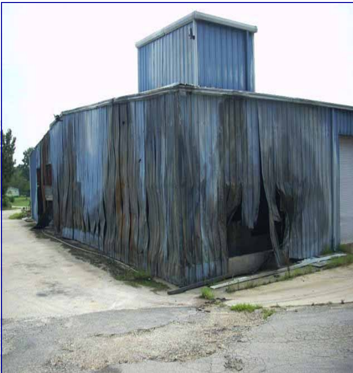
11,200 s.f. main building showing fire damage.
